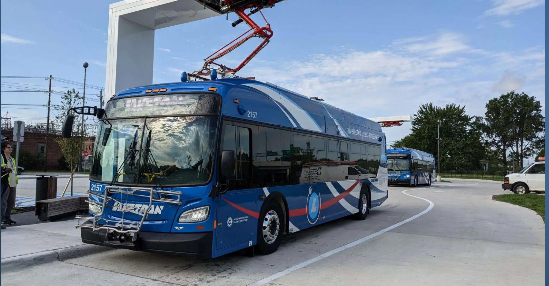
On route ABB pantograph chargers installed by Laketran at a Park-n-Ride location.
